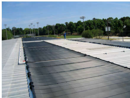
Jobs that can't be outsourced! Tablerock Technologies installs solar panels atop the James Island Recreation Center.
